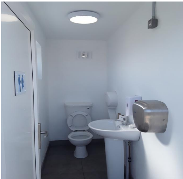
2. The unisex toilet unit.
